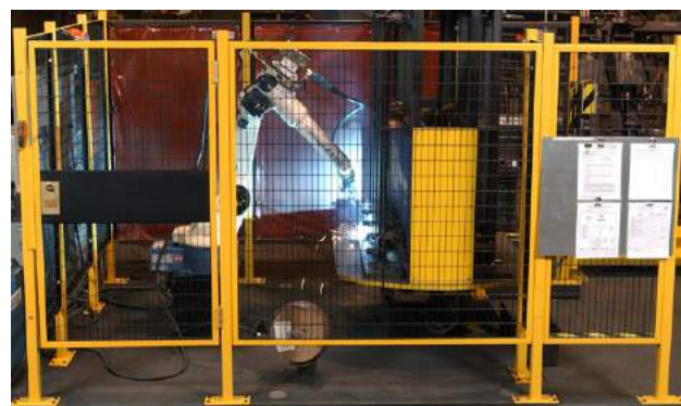
Figure 11: Perimeter fencing for an industrial robot
